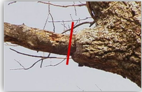
Figure 8. Do not cut into or otherwise damage the branch collar or woundwood growing around the dead branch.
